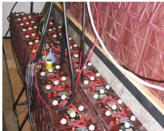
▲ A battery bank
